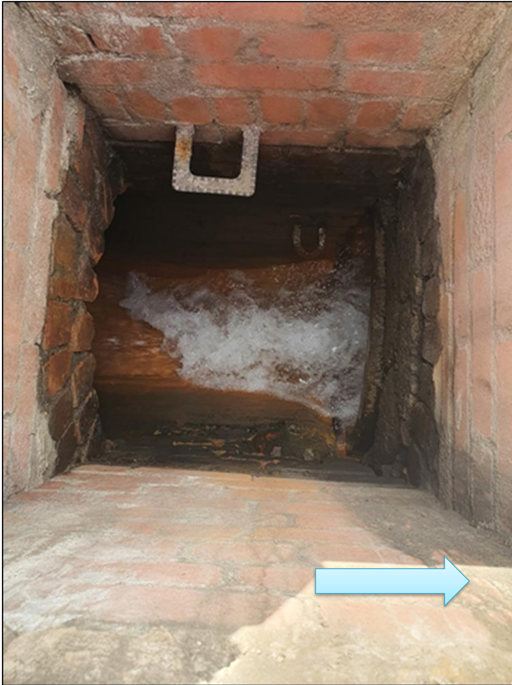
Photograph 4 View of inside inspection chamber that was blocked during Storm Dennis. Arrow shows direction of flow of water. Water is flowing freely and unobstructed. (June 2021)
